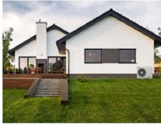
Air Source Heating
